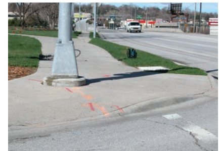
Poor Sidepath Intersection Design. Top: Ramps are narrow and located off line from a bicyclists normal path, creating a potential hazard. Above: The base of a signal mast arm obstructs the logical path through the
