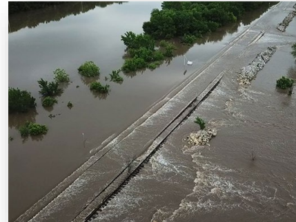
Flooding on BNSF Arkansas City Subdivision May 2019
