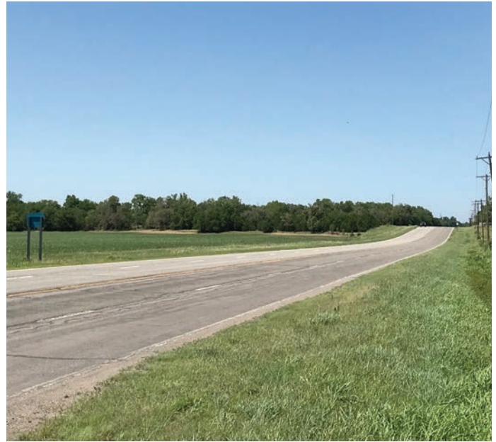
Phase 2 projects include completion of a Hydraulic sidepath from 45th to 69th.
