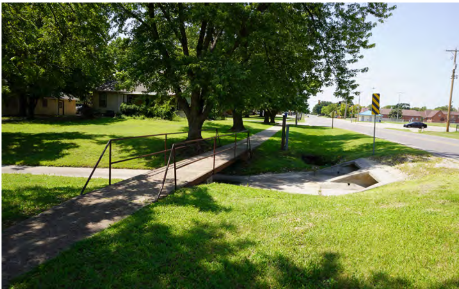
11 / A pedestrian bridge spans a large, concrete drainage channel between 3rd and 4th along Ross Ave.
